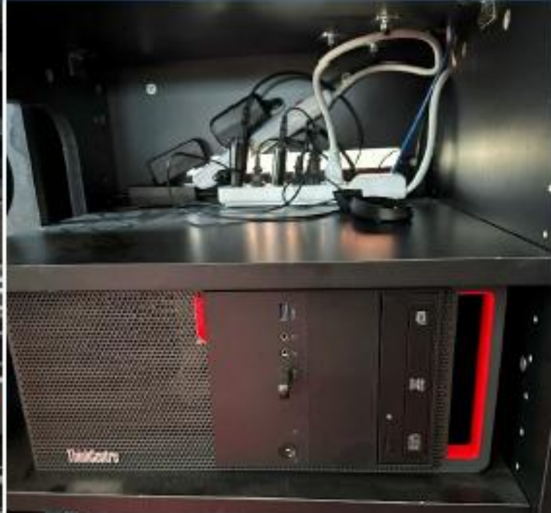
Board room 232: Existing rack 2
